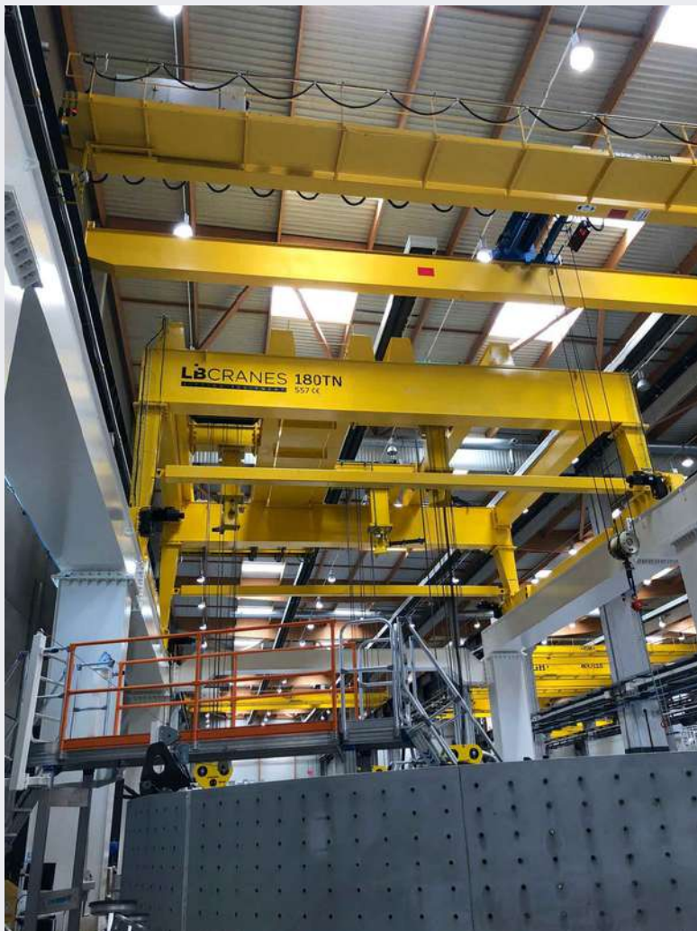
180Tn process crane.
