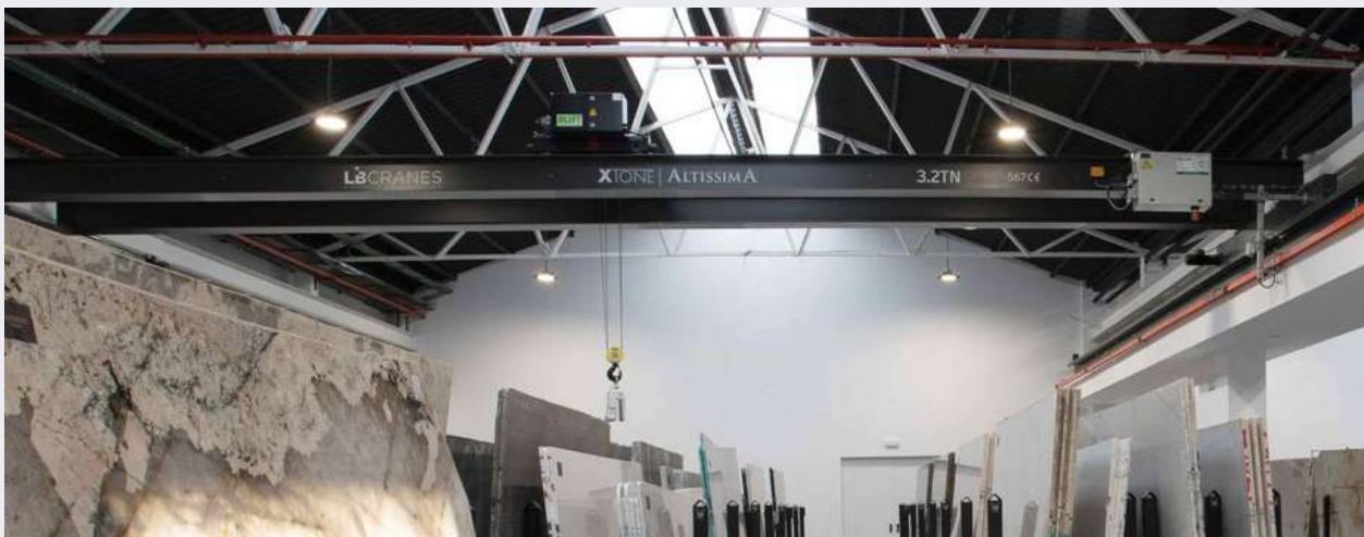
3.2Tn double-girder overhead crane
