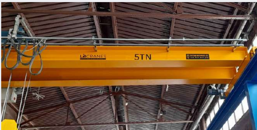
5Tn double-girder overhead crane.
