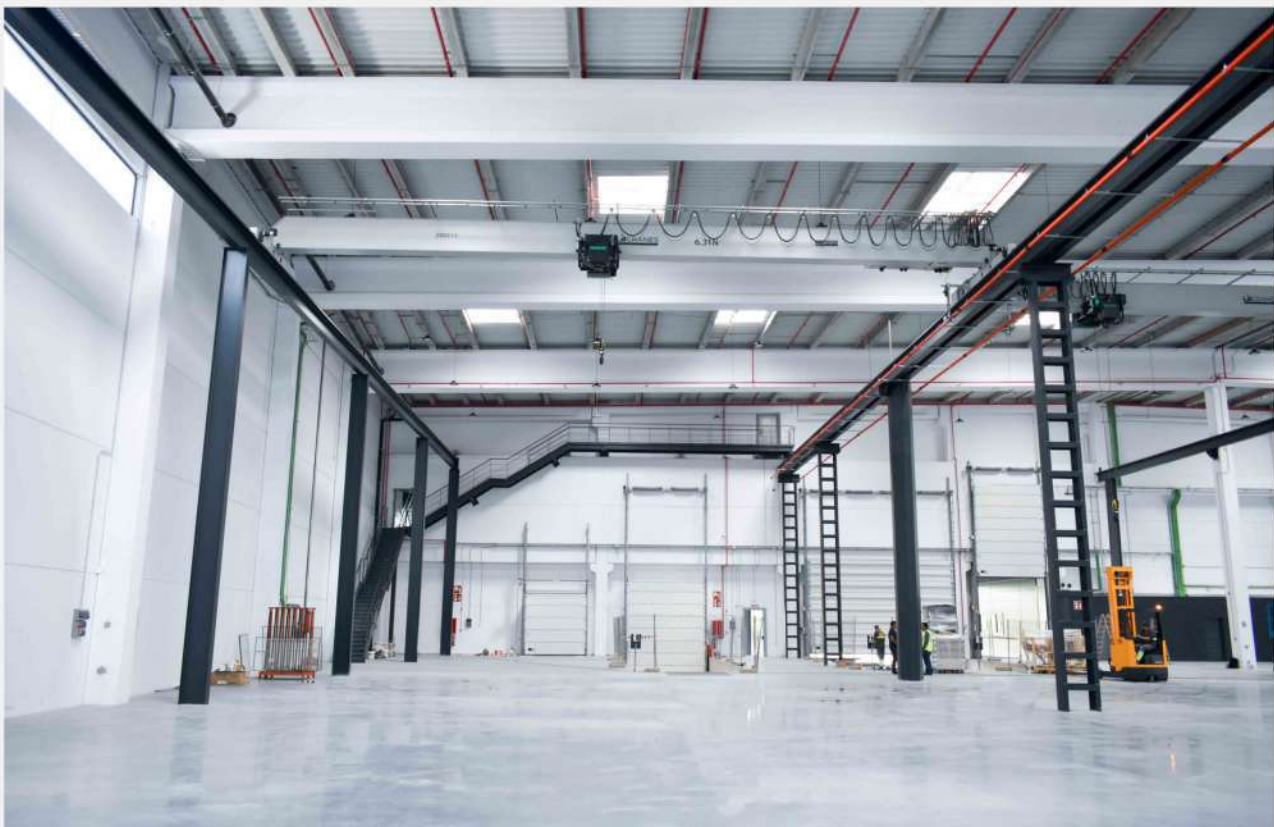
Monorail overhead crane 6.3Tn, undergoing a maintenance check.
